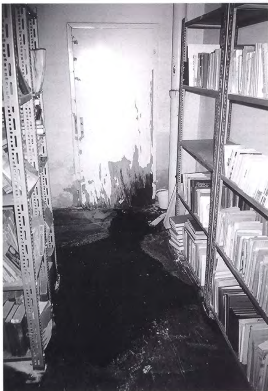
Serious water damages in the main library of Skanderaj located within the House of Culture.
