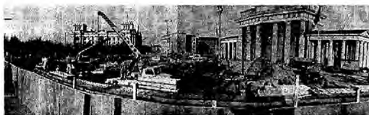
The concrete wall being put up in front of the Brandenburg Gate (20.11.61)
