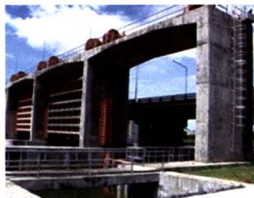
Remote Control System for Water Gate
