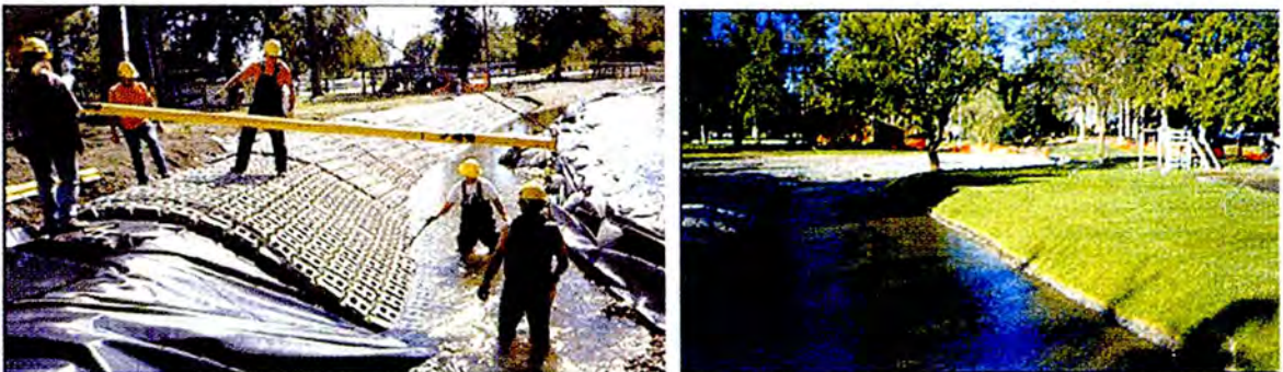
A coffer dam was constructed down the middle of the channel to divert flow away from work area.
